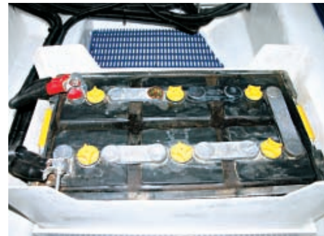
a dedicated start battery, two are house batteries, and one supplies the Northern Lights 12kW generator.) A ProMariner IV 2,000-watt inverter rounds out the standard electrical package. Ocean Alexander representatives say the boat's electrical system is ABYC compliant.
