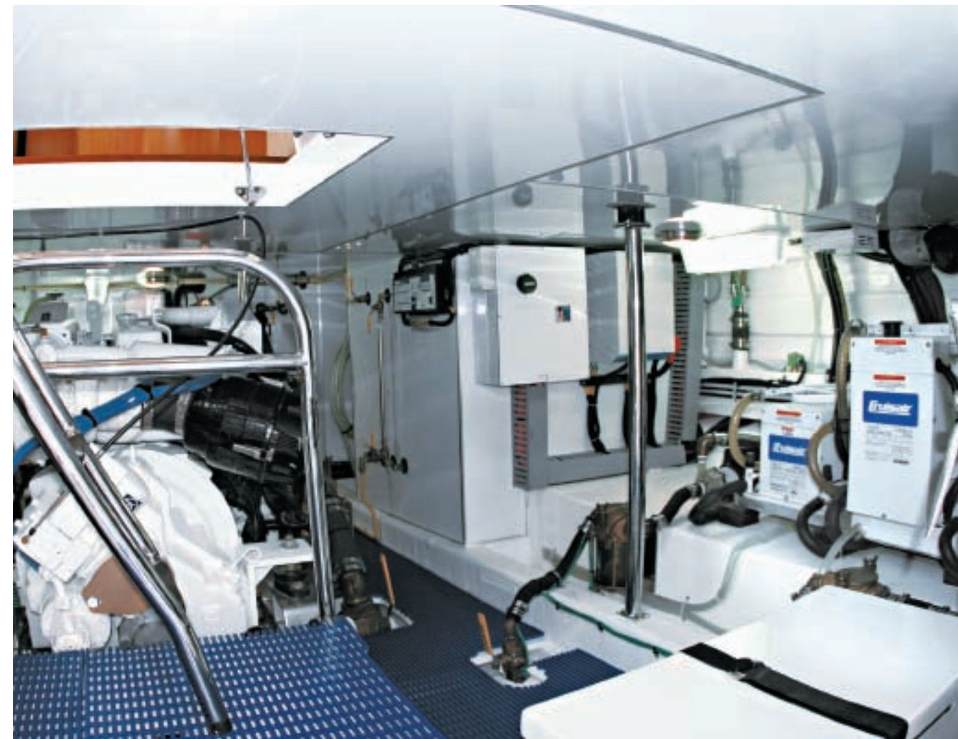
Above: The tidy engine room as viewed looking forward from the lazarette door. The Heronrib flooring provides good footing but is tough on the knees if you're wearing shorts. Right: The heavy fiberglass battery boxes are fixed to the hull and provide excellent containment for battery fluid. The boxes have fiberglass tops that are secured by nylon straps.
