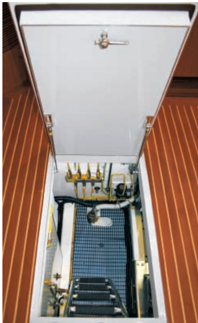
Two heavy hatches provide access to the engine room from the saloon. They are well engineered and are supported with gas struts.
